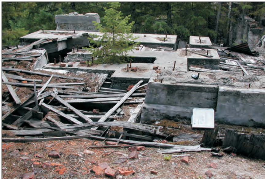
Figure 21. Part of the Red mill foundation at the Republic mine site. Notebook in lower right for scale. View is to the east.
