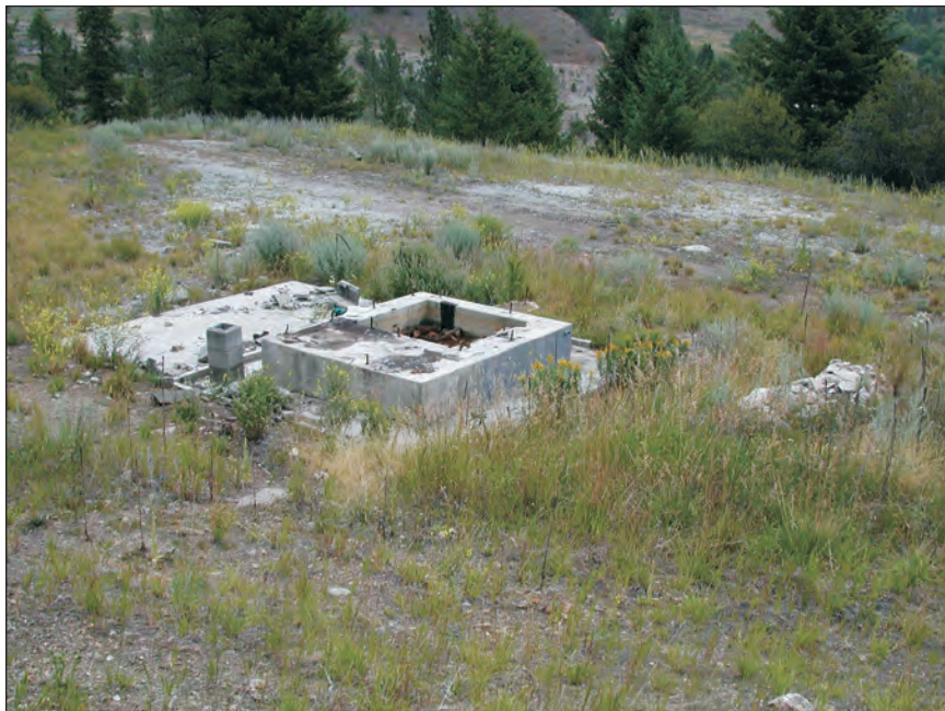
Figure 10. Hoist pad and foundations at the Ben Hur mine site. View is to the north.
