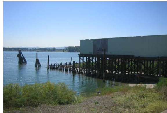
Example of a derelict structure on state-owned aquatic lands Photo: DNR staff.
