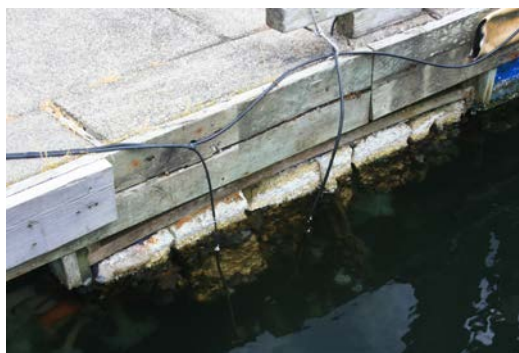
Exposed foam on dock used for floatation Photo: DNR staff
