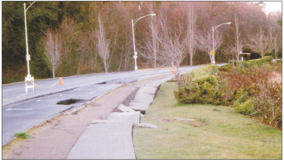
Figure 24. Lateral spreads and settlement with localized sand boils along Deschutes Parkway, Olympia. Damage to the parkway was more extensive in the Nisqually earthquake than in the 1965 Seattle-Tacoma quake. Liquefaction-induced lateral spreading seriously damaged this road on the west side of Capitol Lake. As of this report, ground failures are still occurring and the road is severely damaged along about one-half mile of roadbed. The roadbed is made up of loose fill placed on modern estuarine muds of the Deschutes River, which was dammed in 1956 to form Capitol Lake. Photo by Hank Schasse.
