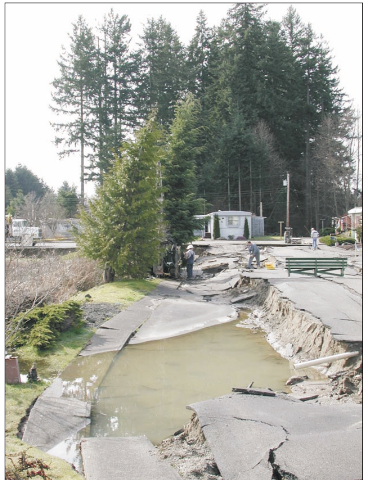
Figure 25. View of the Sunset Lake liquefaction failure about 3 weeks after the earthquake. Fir trees to the left of the failed sidewalk are tilted to the right of vertical, indicating that the toe of this failure has rotated into the lake (to the left of the photo). A drilling rig is located between the two trees, collecting data as part of a research investigation of the failure. Photo by Steve Palmer.
