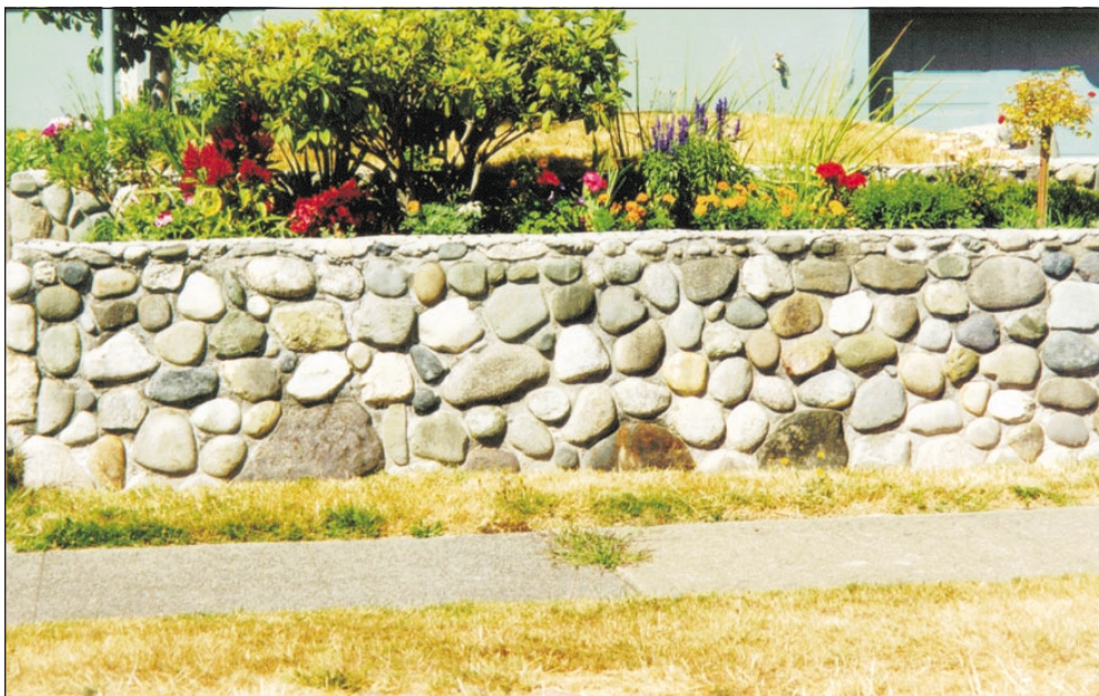
Figure 1. A mortared stone wall in western Washington. Notice that it is thinner and more vertical than the wall in Figure 2. Photo by Wendy Gerstel.
