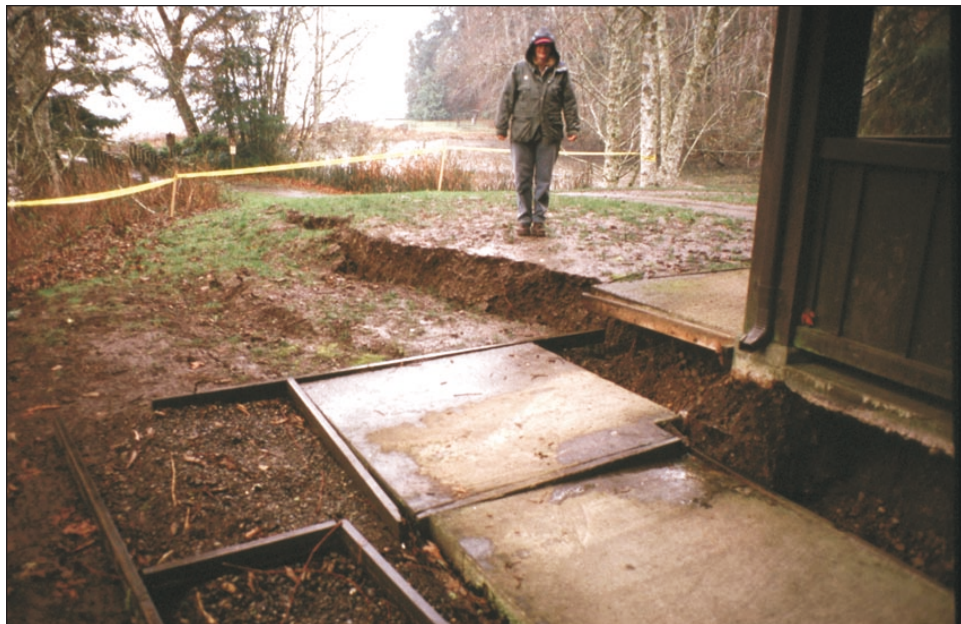
Figure 15. Damage at Tolmie State Park, about 3 miles from the epicenter. Karen Rollman, Park Ranger, looks at a lateral spread at the northwest corner of the kitchen shelter. The shelter, which was constructed on fill, was damaged beyond repair. The concrete foundation pillars supporting the shelter rose buoyantly about 2 inches, and the road and bridge approach leading to the shelter were damaged by numerous ground cracks. Photo by Pat Pringle, March 1, 2001.
