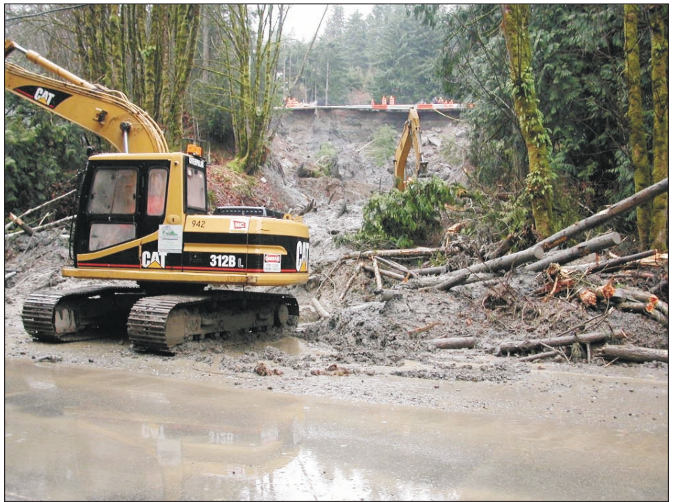
Figure 22. Landslide on U.S. Highway 101 northwest of Olympia. The north lane of the four-lane roadbed liquefied and slid down a ravine. The toe came to rest on a frontage road (foreground). The slide volume is estimated at about 18,000 cubic yards. Photo by Karl Wegmann.
