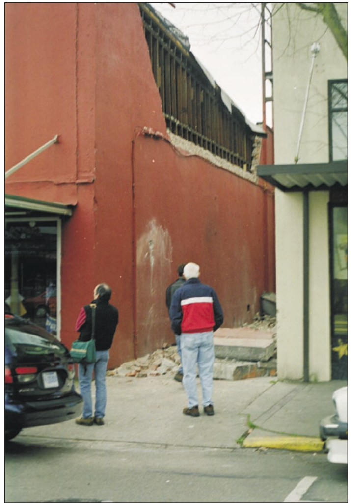
Figure 18. Damage to the Skookum Bay Outfitters building on Capitol Way in downtown Olympia. The chunks of masonry fell right where the UPS delivery truck usually parks at the time of day the quake happened. Photo by Josh Logan.
