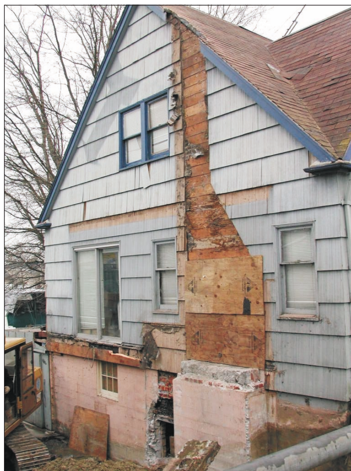
Figure 14. Chimney topple at a private residence at the south end of East Bay in Olympia. The house was built on fill over estuarine muds. Photo by Karl Wegmann.
