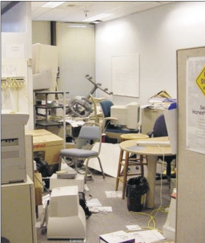
Figure 4. Sixth floor cubicle damage. Photo by Jim Blake, Department of Natural Resources.
