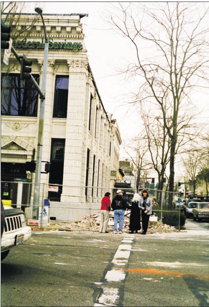
Figure 17. Parapet failure on the south side of the Washington Federal Savings building at Fifth Avenue and Capitol Way in downtown Olympia. Building also pictured in cover photo. Photo by Josh Logan.
