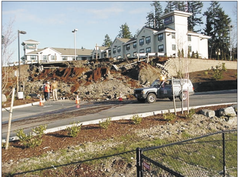
Figure 23. The earthquake-induced retaining-wall failure at Extended Stay America just off Highway 101 in Tumwater. Photo by Steve Palmer.
