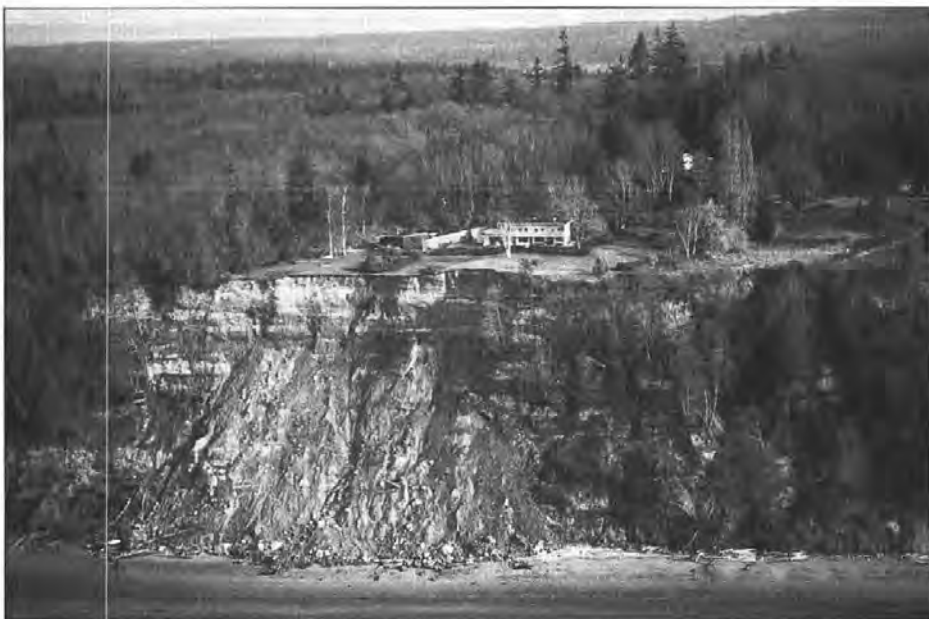
Figure 15. Slide activity such as this in the Useless Bay area of Whidbey Island can cause periodic retreat of the bluff edge by as much as 20 feet or so in seconds. During this recent slide, a portion of the fence in front of the large house was lost. Such episodes commonly are preceded and followed by decades of little erosion, making estimates of average bluff retreat rates potentially meaningless. In this location there are multiple impermeable silt layers that perch water, in contrast to conditions like those at Scatchet Head (Fig. 14), where water is concentrated above one impermeable "perching" layer. Slides here can be triggered by an abundance of water (as in the December/January storms) or by wave erosion at the base of the bluff. A rainstorm may simply be the "last straw". In many locations around the sound, water from winter rains is accumulated inland of bluffs and may cause landslides to occur months later as it slowly migrates toward the bluff. In the mid-1970s in the Golden Gardens area of Seattle, slides occurred well into summer after a series of exceptionally wet winters.
