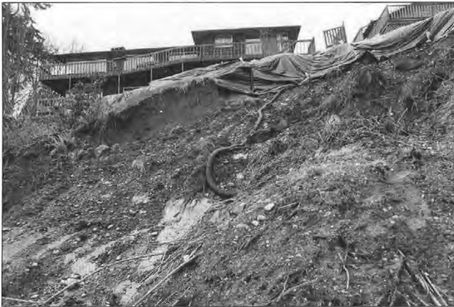
Figure 18. This shoreline home between the Hood Canal Bridge and Port Ludlow lost its front yard during the December/January rainstorms and snowmelt. Bedrock exposed on the beach below the bluff shown in this photo was resistant to wave erosion. However, the glacially polished bedrock perched ground water in the gravelly sand above the steeply sloping contact here. Runoff from rapid snowmelt was apparently funneled down the driveway from upslope development. The area to the left of this landslide (out of view) was probably buttressed by a large maple stump kept alive by sprouts. (The area still farther left also failed.) Glacially compacted silts or bedrock form a barrier to roots and ground water. Where this condition exists in the Puget Lowland, shallow debris avalanches can be common. The overlying permeable saturated soil cannot be anchored to the substrate by the weak toehold of the roots of trees and other vegetation.
