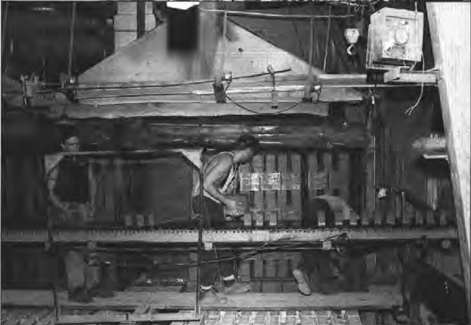
Figure 5. Stacking clay blocks to be sent to the dryer and kiln. The soft bricks move to where they are manually stacked on cars. This is the most labor-intensive part of the process. Once stacked on the cars, the clay blocks are moved along rails through the dryer and the kiln. The Mica plant can produce an unusual near-white brick from the Latah deposit. Because of this characteristic of the clay, the company can also make bricks in a number of light or pastel colors by adding colorants or small amounts of clay of another color.
