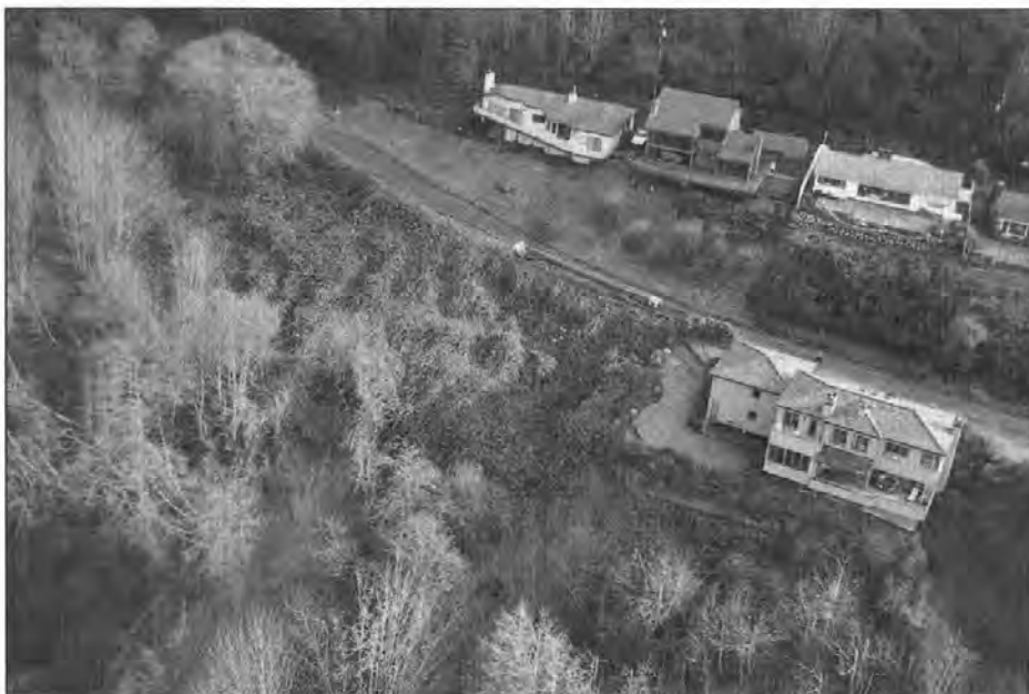
Figure 7. This house in West Seattle (lower right), and a portion of the road that runs behind it, are built on fill, commonly failure-prone when saturated. Note the down-dropped (and previously patched) section of the road between the white signs. Tension cracks start to the left of this area and extend to the right, under the house. Fill material at the lower right corner of the house appears to be displaced. Also note the recent debris flows in the drainage below the road (lower left center of this photo). These may have been caused by excessive runoff onto colluvium and fill.
