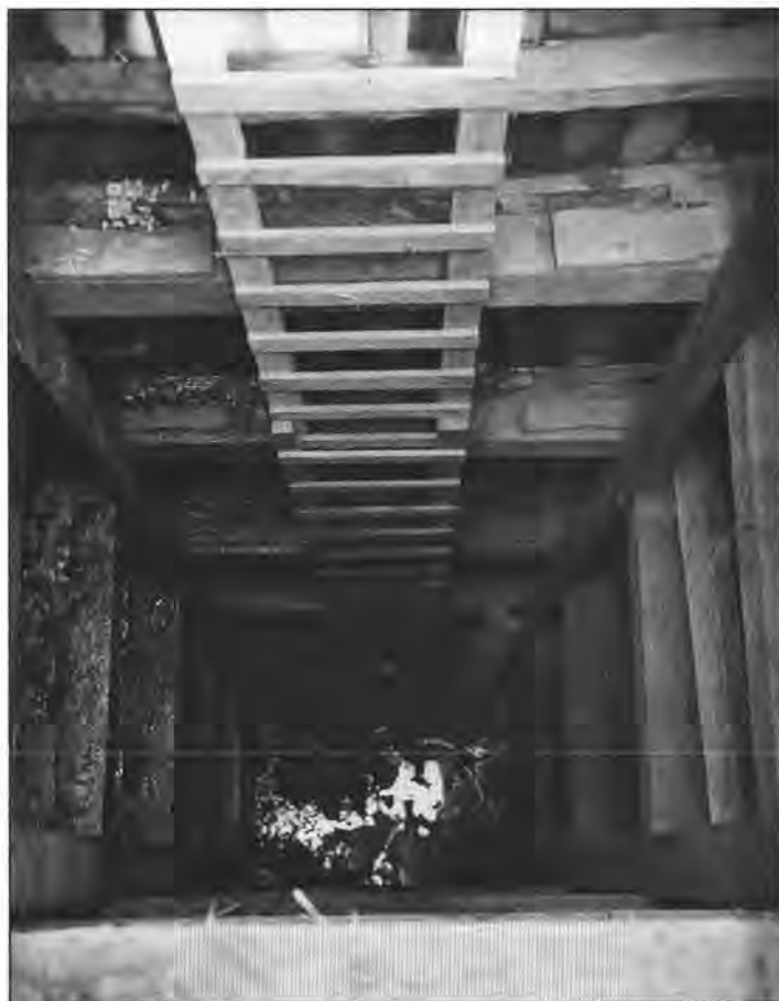
Figure 12. Manhole shaft being excavated, showing waling and access, Madrona Drive and East Pine Street slide (site 16, Fig. 2). (Courtesy of the City of Seattle Department of Engineering.)
