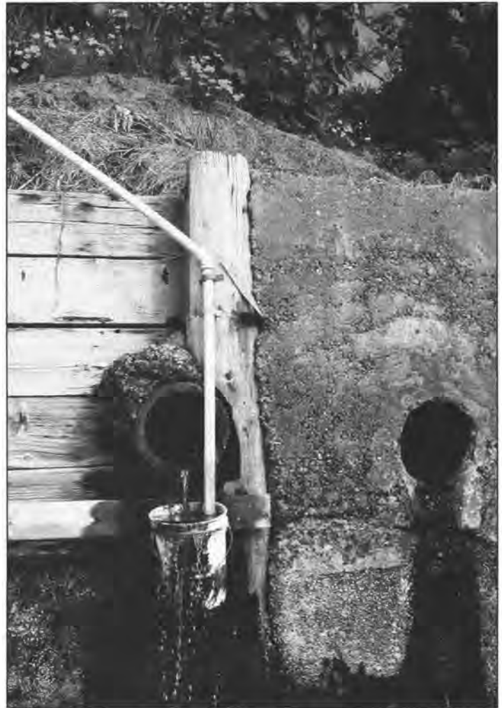
Figure 13. Drain pipe protruding through the seawall at the West Bertona Street tunnel portal. (See also Figs. 1 and 10.) Photo taken September 1994 by S. Evans.
