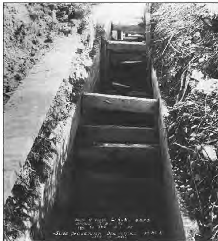
Figure 6. Closeup of slide control trench drain showing protective lagging and bracing timbers, South Dose Terrace and 34th Avenue South slide (site 22, Fig. 2). Trench width approximately 30 inches. Photo taken March 1935. (Used with permission of the Special Collections Division of the University of Washington Libraries, UWNeg#15389.)
