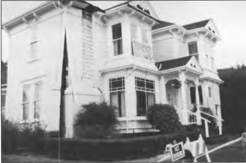
Figure 7. Many houses in Ferndale, CA, sustained severe damage from the earthquakes of April 1992. This house was one of many that lost chimneys. The house in the cover photo was knocked from its foundation.
