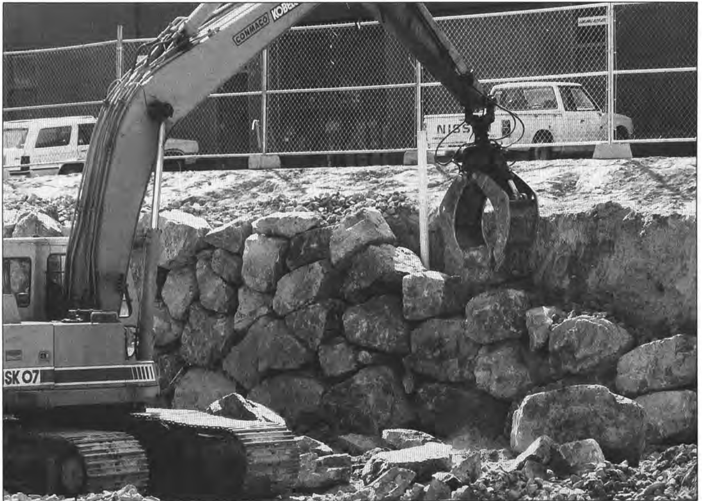
A retaining wall of boulders (or a rockery) under construction in the Seattle area. See related article on p. 3. Photo supplied by Associated Rockery Contractors.
