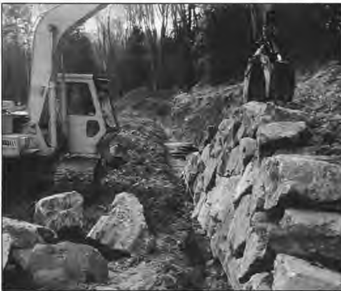
Figure 1A. A rock wall (rockery) being constructed. Photo courtesy of Fred Hackney, Alpine Rockeries, Woodinville.
