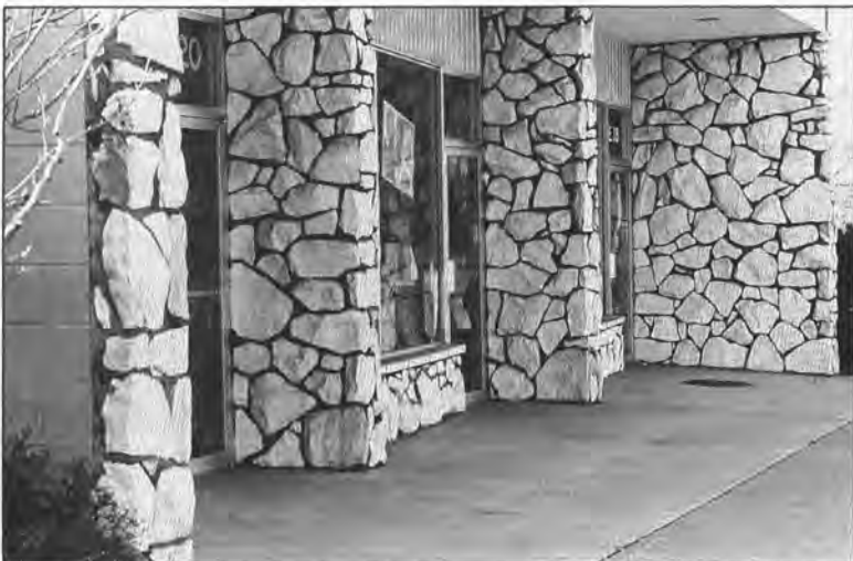
Figure 11. A rubble wall that consists of irregular pieces of marble, each of which has one essentially flat face.
