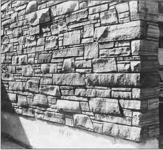
Figure 2. A sandstone wall consisting of rectangular blocks of ashlar laid randomly in courses.
