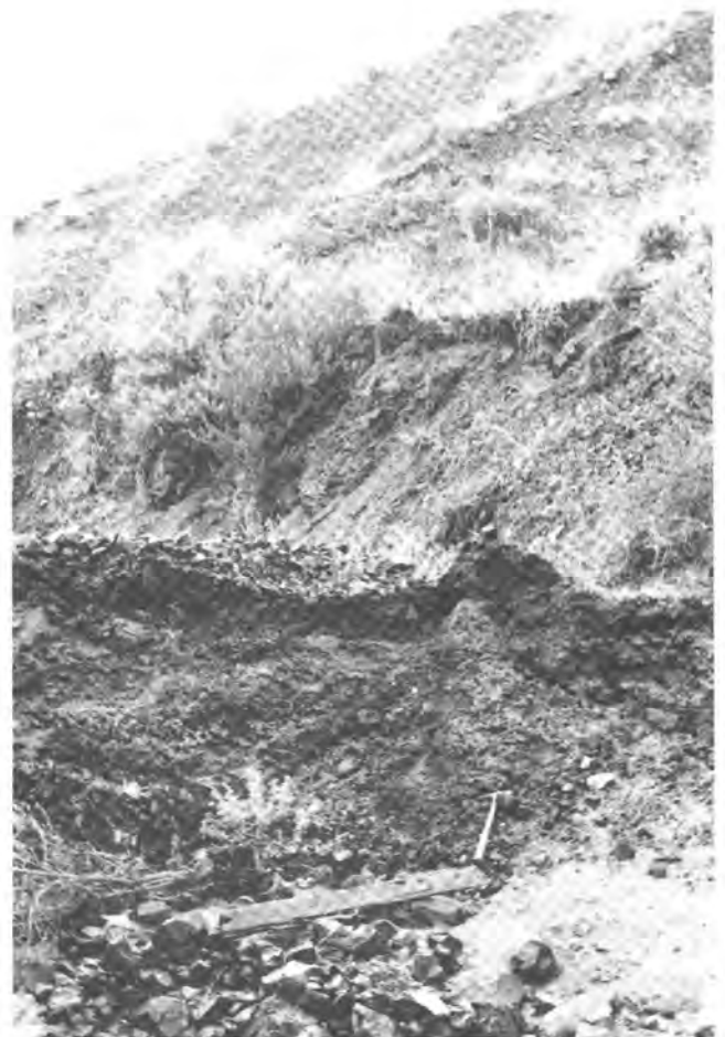
Figure 7. An alluvial terrace in the canyon at the toe of the deep-seated failure. The present canyon floor is several feet below the terrace (at hammer level), indicating that the landslide toe dammed the canyon and was subsequently breached.
