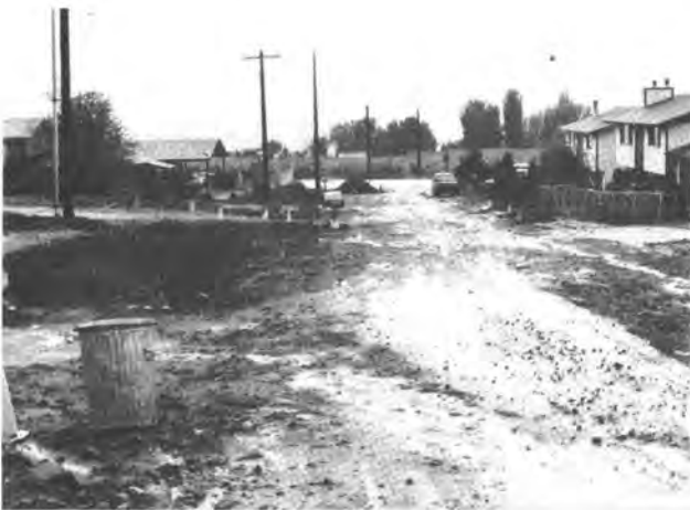
Figure 9. Erosion along a street on the Canyon B alluvial fan. State Highway 28 is in the background. Floodwaters were nearly 3 feet deep at the lower end of this street.
