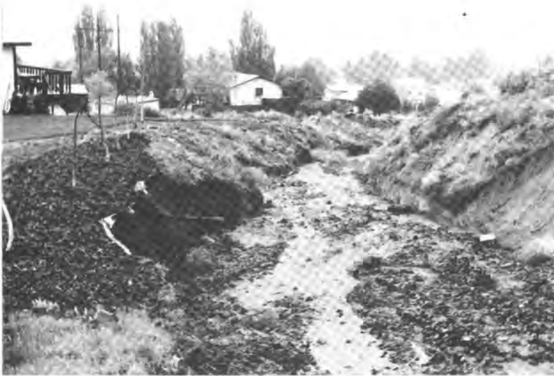
Figure 8. Stream-bank erosion in the residential area located on the Canyon B alluvial fan. Note the unsupported pipe in the bank on the left, slope failures on the right.
