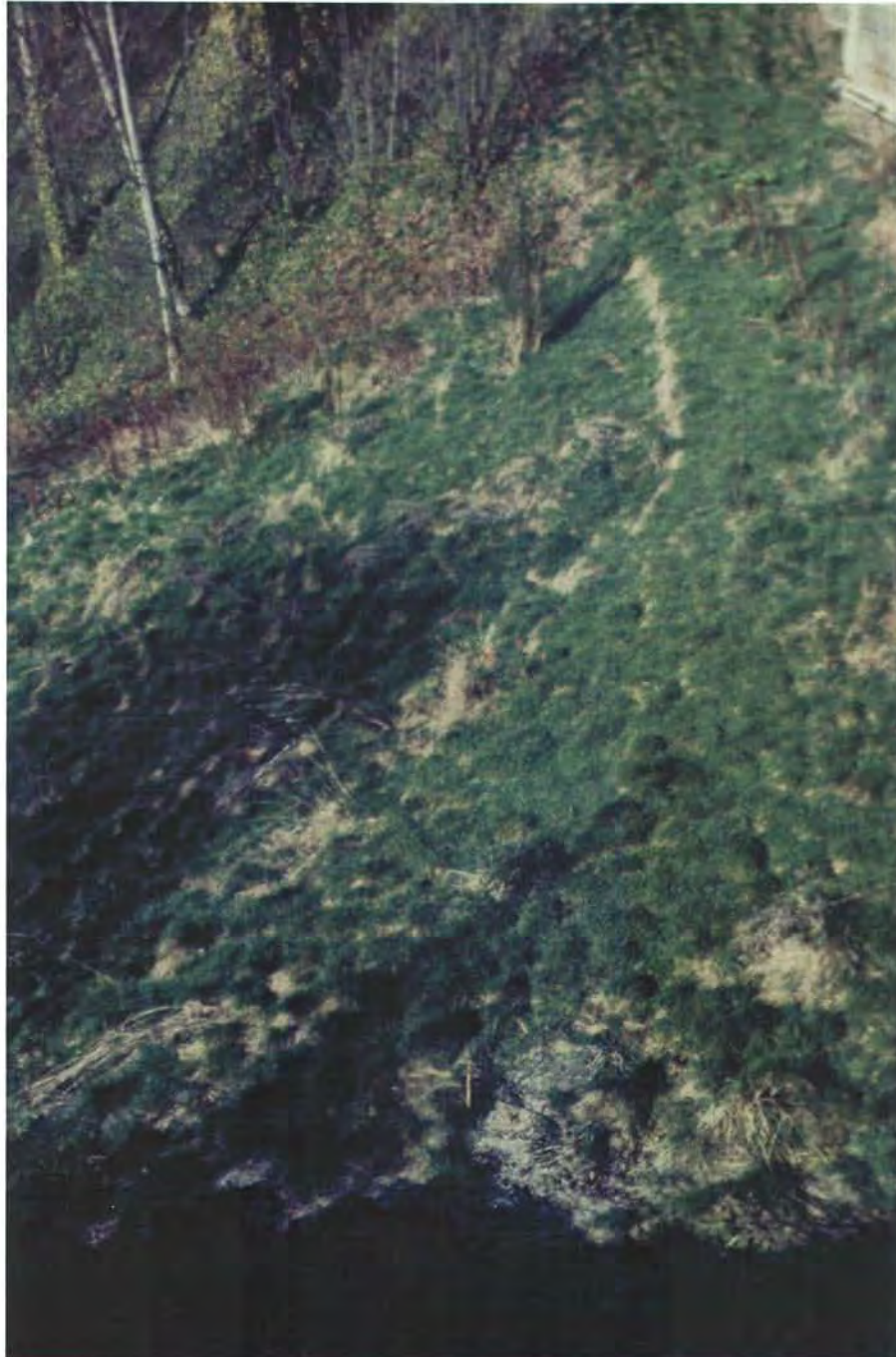
Figure 7 Photograph of the headscarp of a landslide failure that occurred on the slope below the retaining wall west of the GA building. This failure occurred sometime between the fall of 1992 and the spring of 1993.
