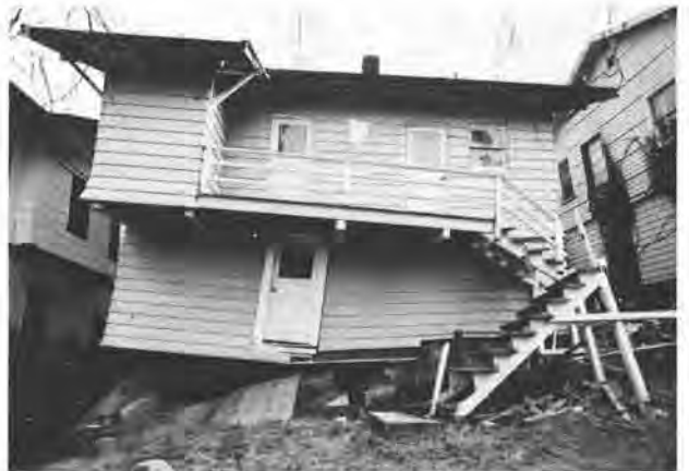
FIGURE 3.—Landslide effects in the Madrona District.
