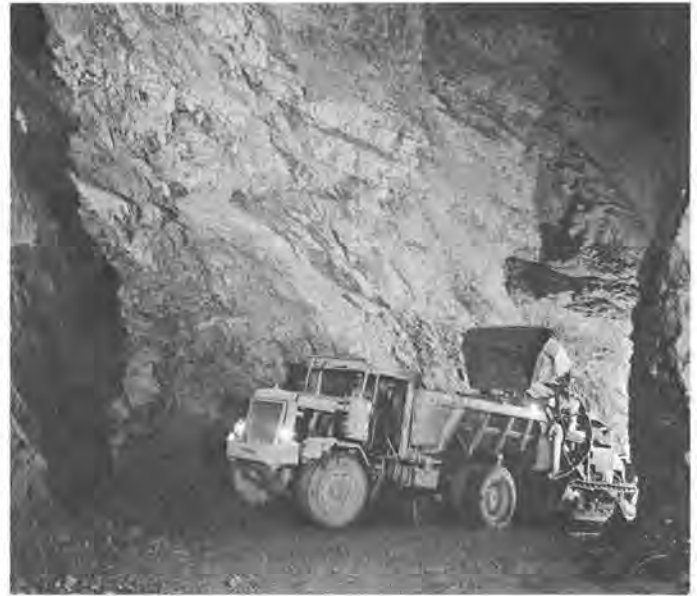
Loading of a 12-ton truck by a front-end loader underground in the Pend Oreille Mines & Metals Co. mine at Metaline Falls, Pend Oreille County. (Photo courtesy of Pend Oreille Mines & Metals Co.) Figure 46.
