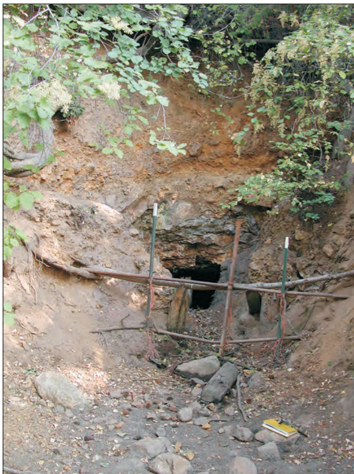
Figure 13. Haulageway portal, lower adit site, at the Sonny Boy mine. Water ~2 feet deep is impounded behind the colluvium dam (notebook for scale). View is to the southeast.
