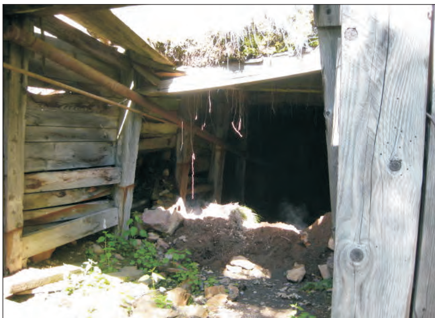
Figure 22. Overburden collapse at the adit portal, June 2010.
