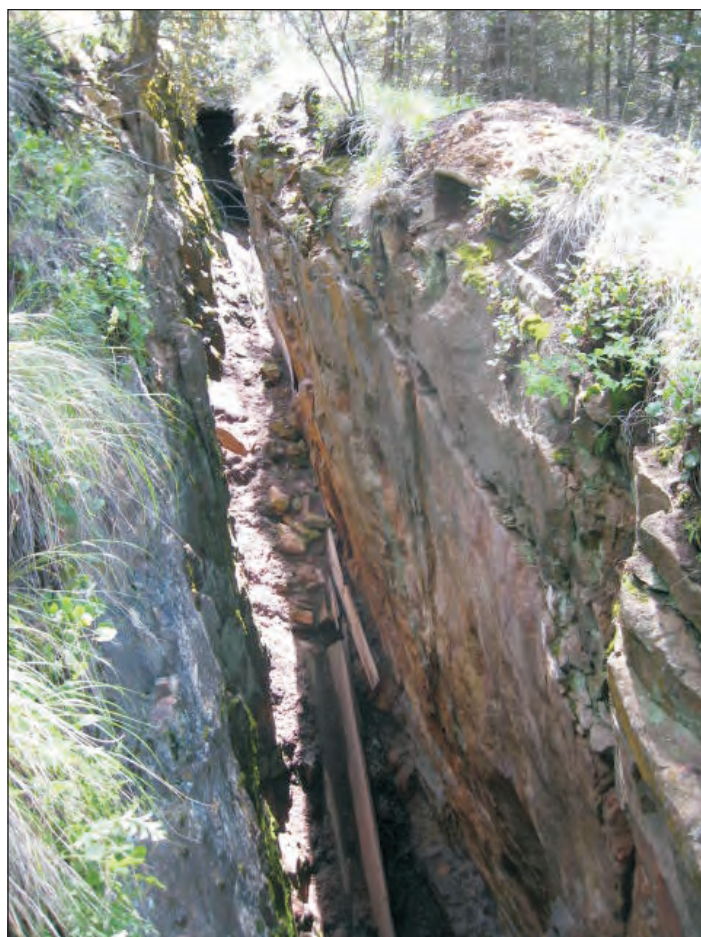
Figure 10. Open stope at the Sonny Boy mine is approximately 30 feet deep at top left by 7 feet wide. View is along strike to the southeast.
